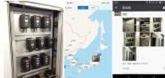
日本熊谷化纤 Chemical Fiber, Kumagaya, Japan
