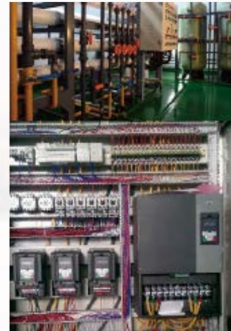
恒压供水, 保障万千 用户的用水需求 Constant Pressure Water Supply the Water Demand of Thousands of Users
